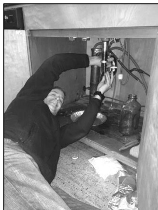
Tony Richards fixing the cracked trap under the kitchen sink
