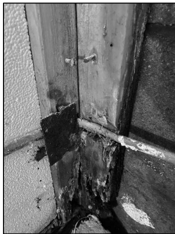
Wet rotted structural elements in bedroom D
