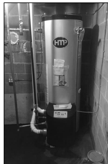
One of the new propane heated water tanks
