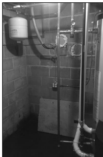
The new water filtration system
